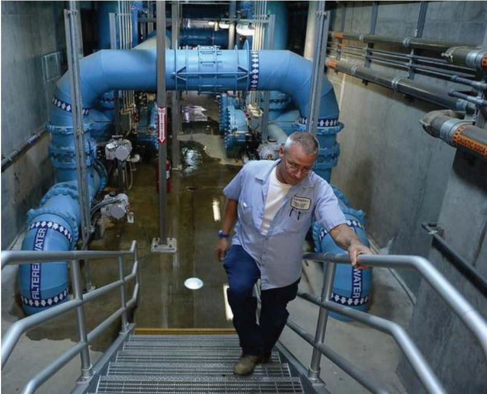
In September 2013, plant operator Brad Hoagland inspects equipment in the filter gallery at the city of Fresno's water treatment plant in northeast Fresno. (MARK CROSSE — THE FRESNO BEE)
